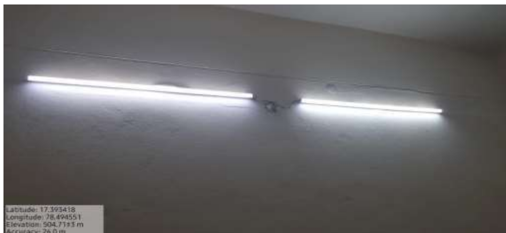
LED BULBS: Energy conservation measures
